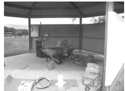
"Ed Wolski of Scamander works on the brickwork for the fitting of the Cornwall Park BBQ"
