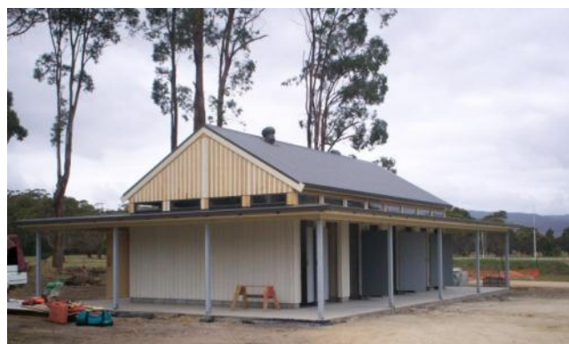
A work in progress. Toilet & shower block at the St Marys Recreation Ground.
