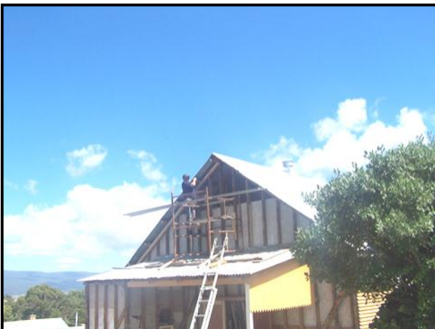
St Helens builder, Glenn Ihnen, begins the re-cladding of the Cornwall Hall
