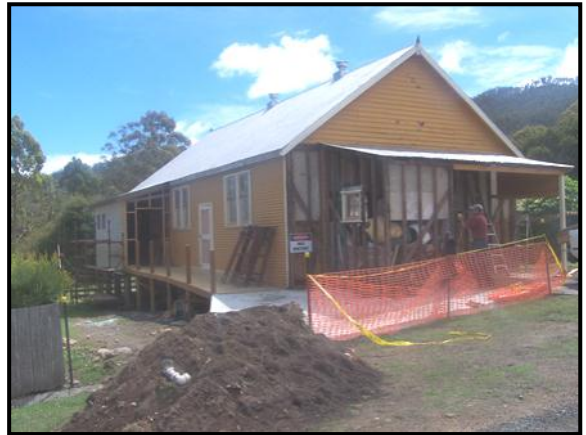
Cornwall Community Committeeman, Graeme Hayes, prepares the Cornwall Hall for a face lift.
