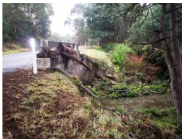
Debris build-up on Margison's Creek bridge.
