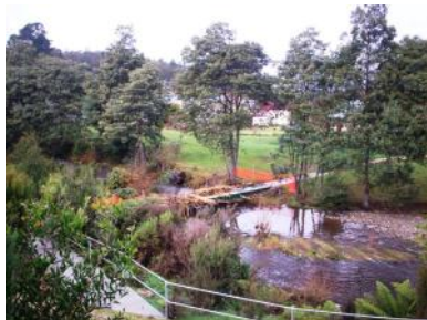
Wombat Walk new footbridge with damaged railing.
