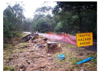
Margison's Creek Bridge wash out.
