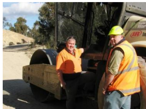
Leigh Daniels about to climb into the heavy roller and Ivan Semmens at work on the S Road repairs.
