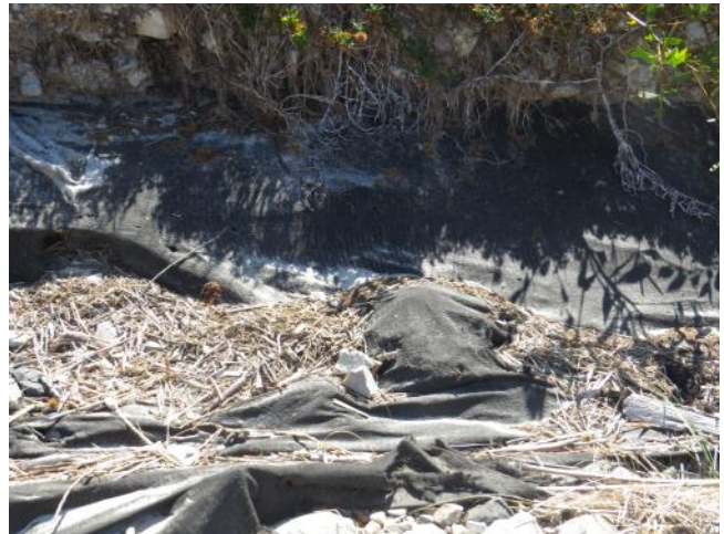
Rock wall has collapsed, exposing the black geo cloth
