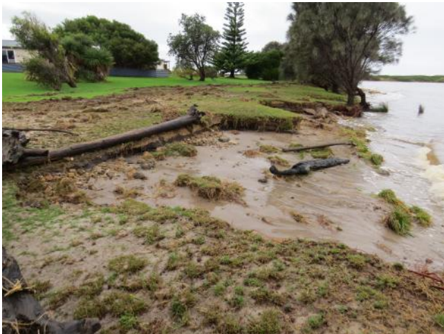
Serious Scamander foreshore erosion
