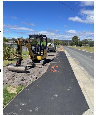
BODC works trainee Sophie and works team member Murray working on the Young Street footpath.
